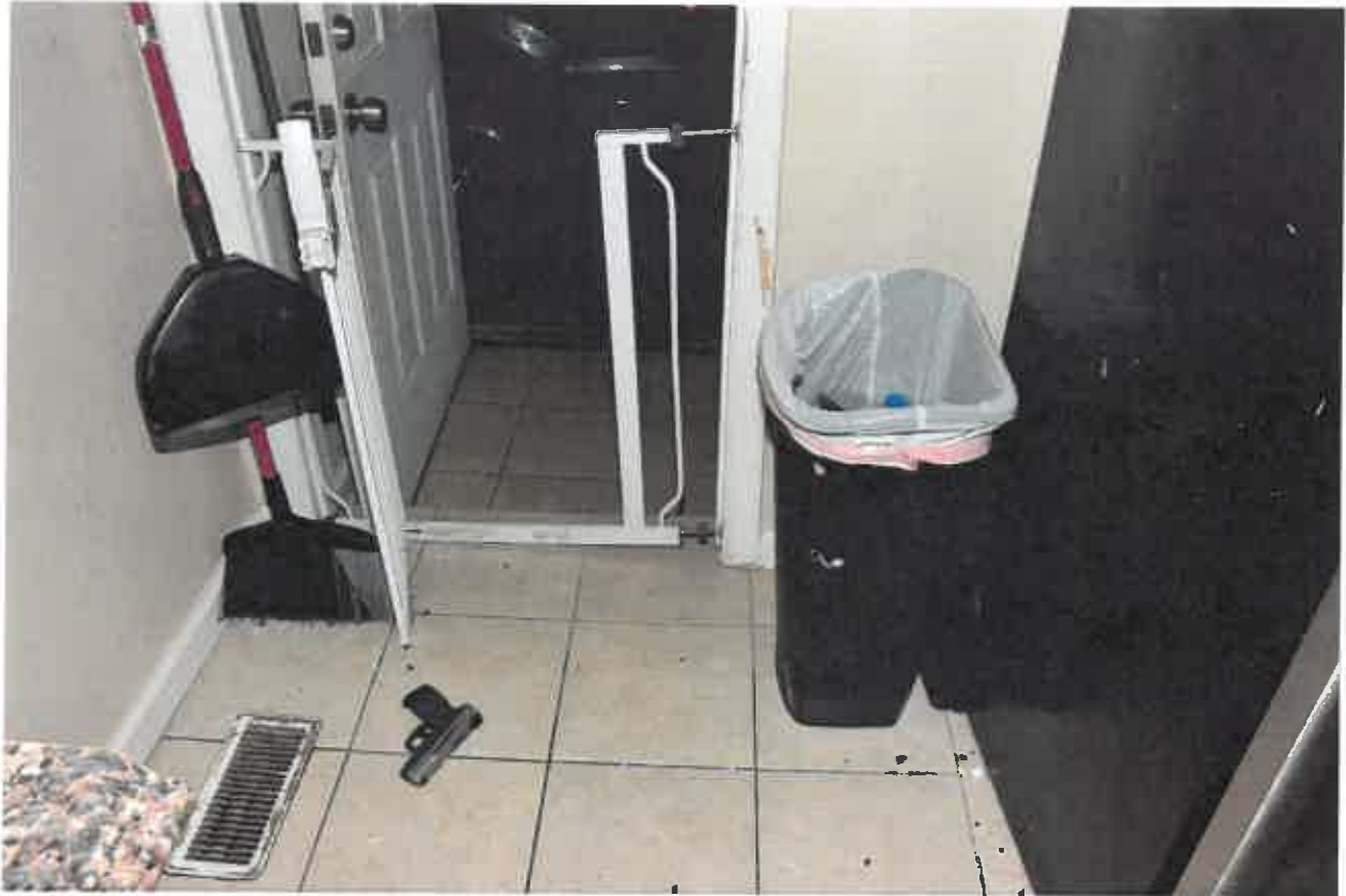
(View of the side door from the kitchen and the area that Mr. Sanchez-Jimenez fell)
