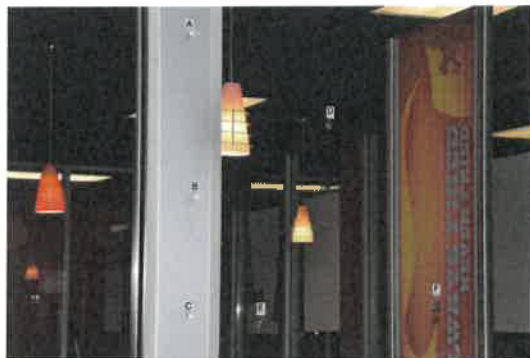
Exterior windows on the south side of the Burger King facing 45 th Avenue. Markers A - F show bullet defects.
